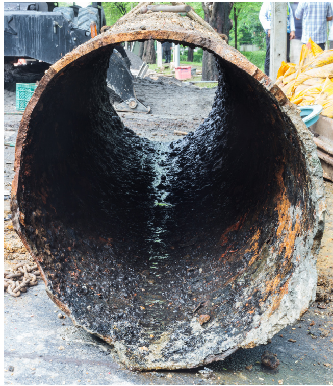
DN 700 Cast iron pipe broken by water hammer
