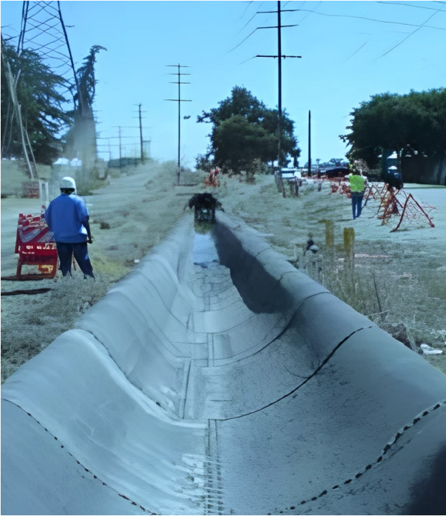
Collapsed pipe caused by vacuum
