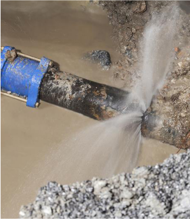
Pipe burst caused by water hammer
