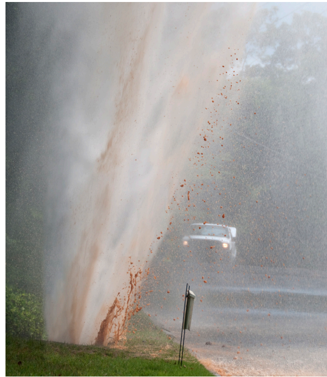
Severe pipe burst which can pose serious health and safety risks
